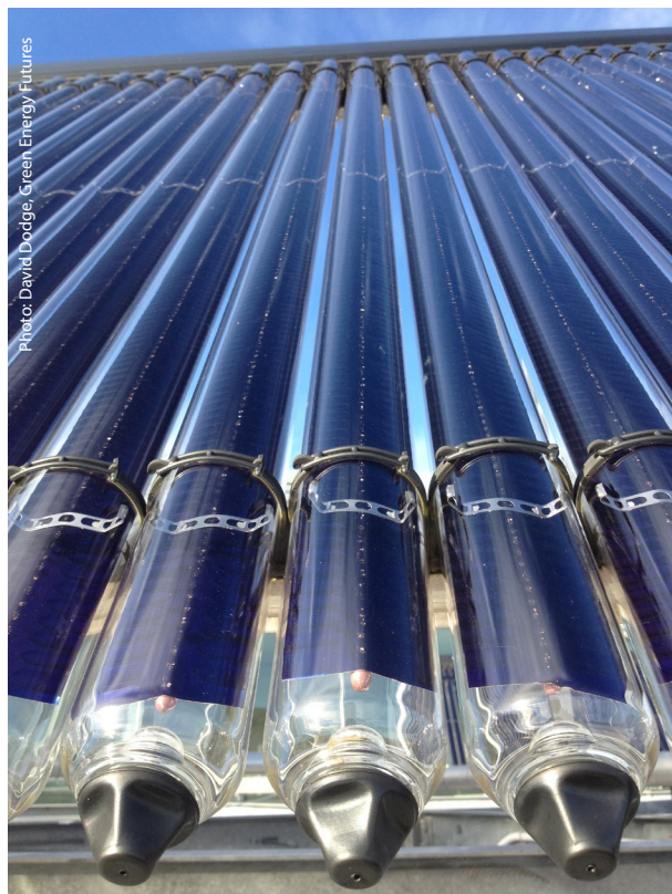
Solar water heating system
