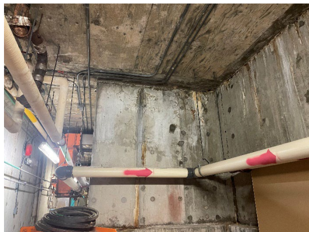
Pool Tank Wall – Spalling and Corrosion
