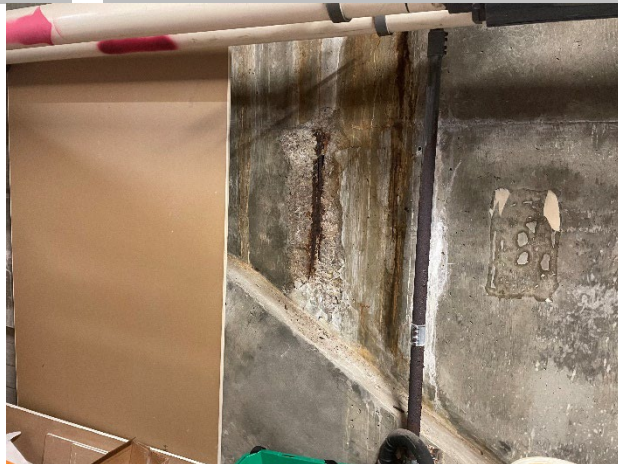
Pool Tank Wall – Exposed Reinforcement
