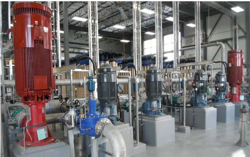
Photo: View of water supply pumps on the main floor, with beige filtration racks in the background.
