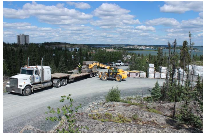
Preparing to begin construction on Yellowknife's new Water Treatment Plant, Summer 2014 (City of Yellowknife Photo)
